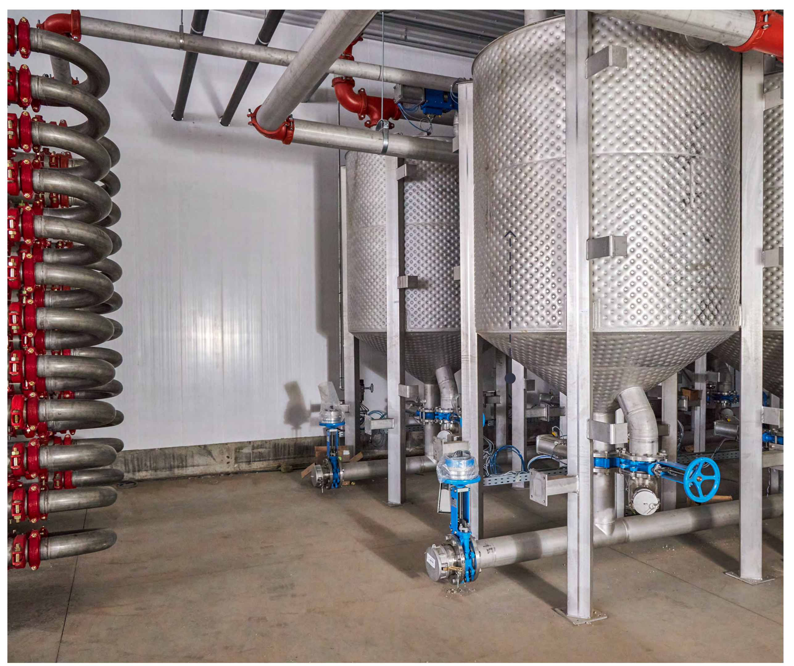
DOUBLE-TUBE HEAT EXCHANGER AND HOLDING TANKS
